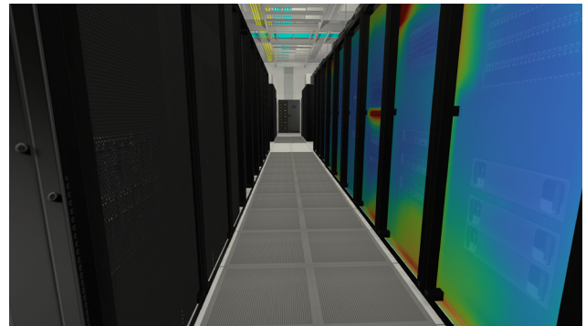
Figure 1: Cadence Reality DC Digital Twin showing simulation results of the cabinet thermal temperature plane
